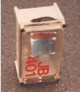
Excessive heat from high current will damage enclosures
