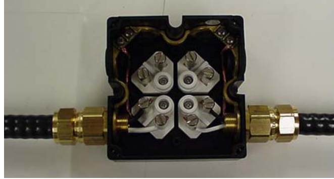
Conductors must be terminated at Ex-e connections
