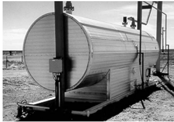
The inside of a vented storage tank is typically Zone 0.
