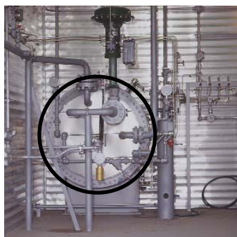
Gas detectors in process plants detect the presence of volatile vapors.
