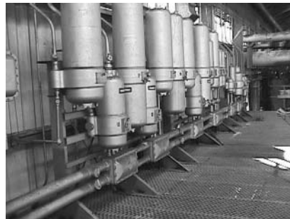
Most hazardous areas located indoors were classified as Division 1. (Old-style motor starters have been replaced by EBM's.)
