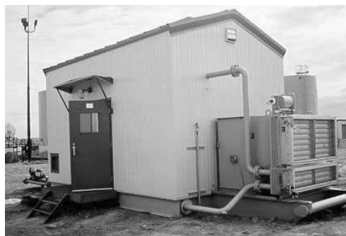
Many skid platforms are not manned and are classified as Zone 1.
