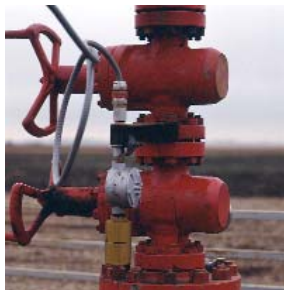
Wellhead and gas detector.
