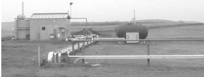
Remote pumping stations should have gas monitors installed to detect gas leaks.
