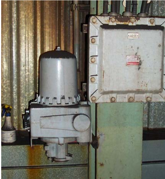
Good housekeeping measures of eliminating dust deposits are important in Class II locations.
